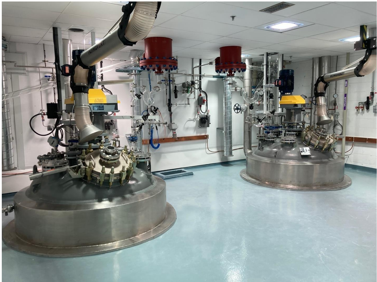
Photo 1 Caption: Plant 3 Reactor Suite, 4000L and 3000L Glass-lined Reactors
