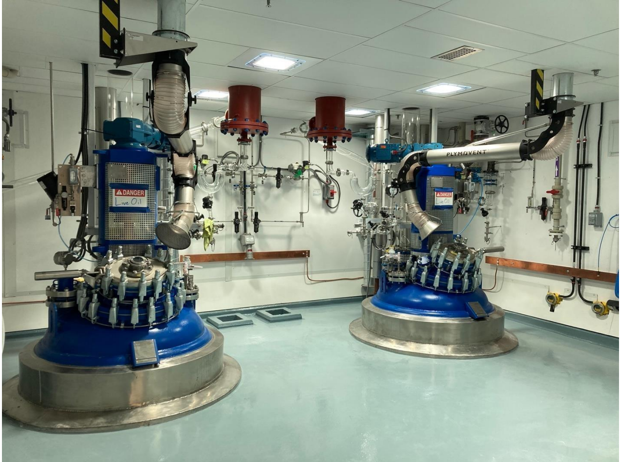
Photo 2 Caption: Plant 3 Reactor Suite: 2 x 2000L Glass-lined Reactors
