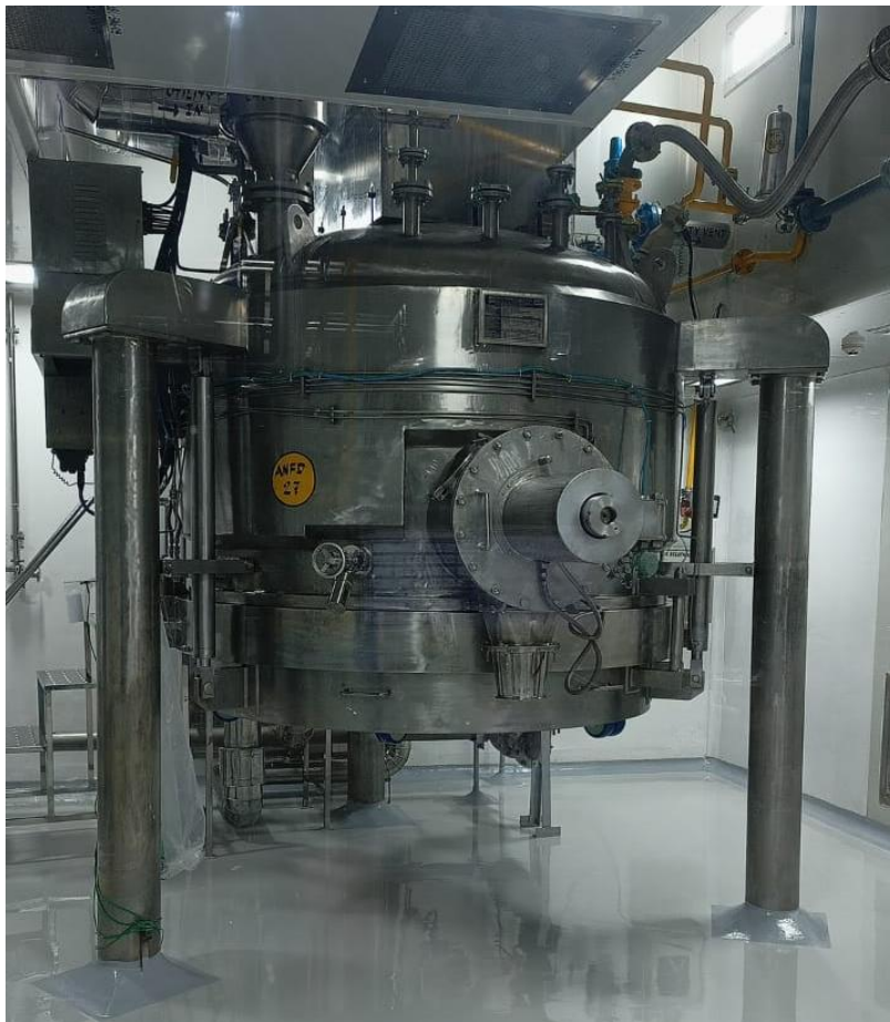
Agitated Nutsche Filter Dryer (ANFD) in Pharma Area, Digwal H Block
