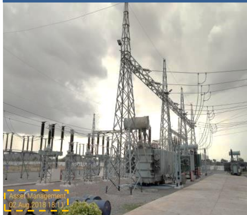
33 kV line connecting with the sub-station
