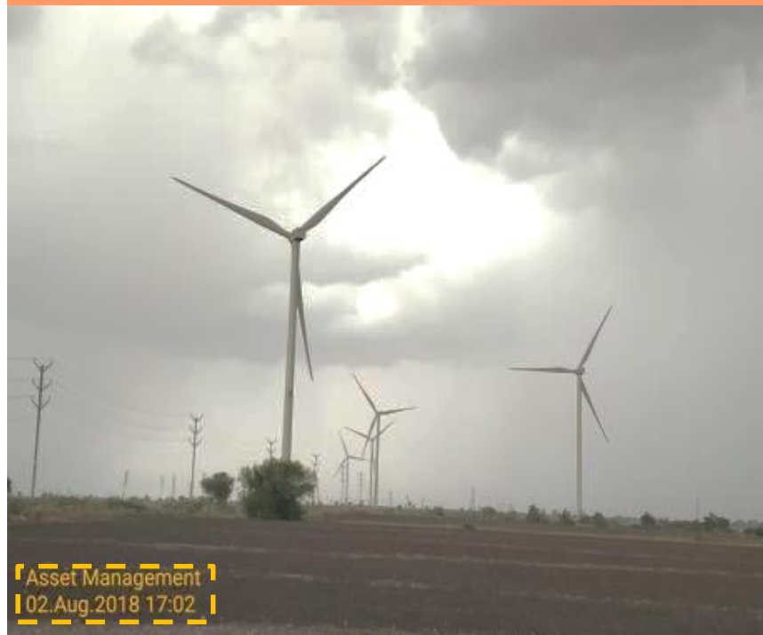
Operating wind turbines along with 33 kV lines
